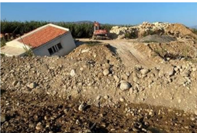
Photo 6 The area of construction work for the biological waste treatment facility of Rethymno, on the nesting beach. (July 2021)
